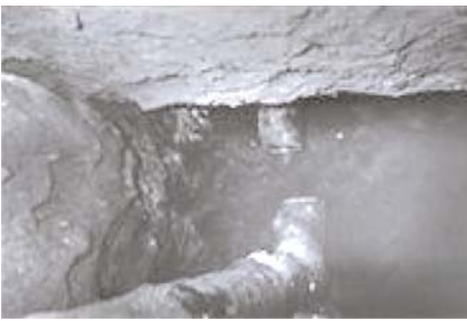
Figure 1 Failed joint connection following the Loma Prieta Earthquake. National Information Service for Earthquake Engineering photo.
