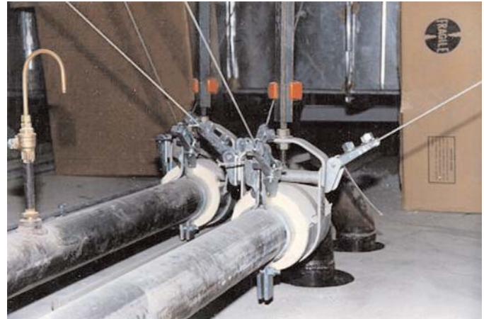
Figure 3 Cable stayed bracing. Photo from Mason Industries, Inc.
